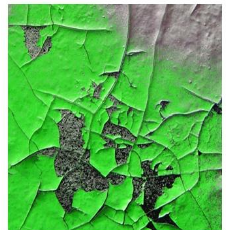
Underlying paint shows severe cracking due to solvent attack from the graffiti
